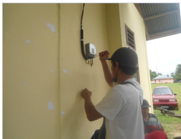
Fig. 4. Increasing Electricity from 900 Watts to 4500 Watts
